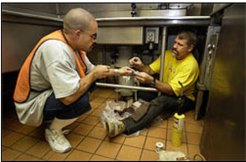
Inmate Mario Herrera, left, helps plumber Richard Williams install a new kitchen faucet at California State Prison, Sacramento.
