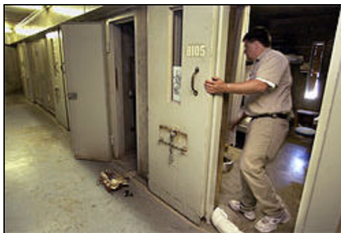
Plumber Brian Coughran changes a water valve in a cell at California State Prison, Sacramento, where the sewage and water system has frequent breakdowns and vandalism. Prison plumbers are classified as public-safety workers, making them eligible for fatter pensions and disability benefits.
